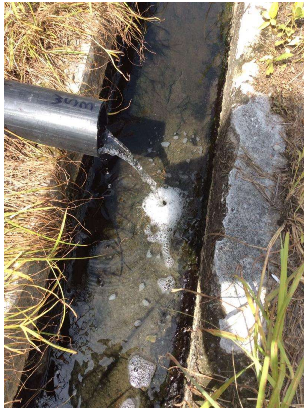
DHS Overflow Part
